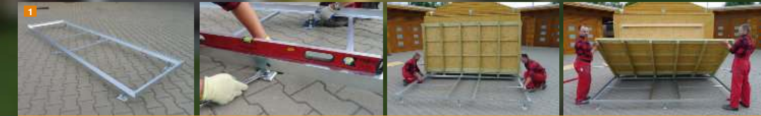
Installation of the foundation frame: put the kiosk onto the first frame, install and level the second frame. Done!
