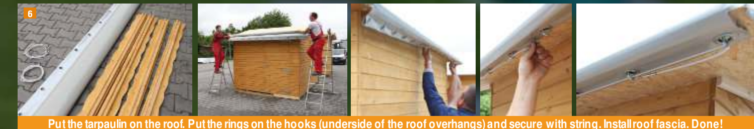
Put the tarpaulin on the roof. Put the rings on the hooks (underside of the roof overhangs) and secure with string. Install roof fascia. Done!
